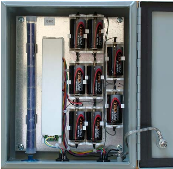
Photograph of battery holders
